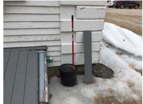
Figure 49 – Asphalt roll roofing on bulkhead covered with failing v-groove pine.
