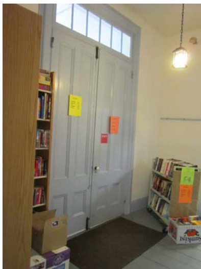
Figure 52 – double doors from vestibule to original hall match fixed exterior doors at northwest facade
