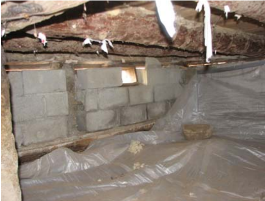
Figure 41 – Infill masonry does not contact building timber sill above, sparing the building frame from frost related damage.
