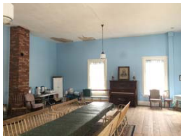
Figure 55– Mason's Meeting Room showing abandoned chimney and extent of damaged ceiling plaster
