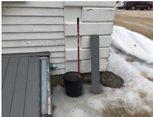
Figure 43 – Original granite pier at north building corner remains. Original masonry has been removed and a small basement space is accessed via bulkhead in need of repair.
