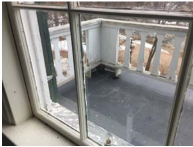
Figure 48– false corner posts at balustrade on entry canopy roof limit penetrations through EPDM roofing
