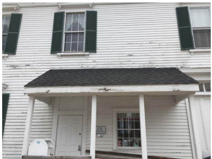
Figure 47– Water damage at porch fascia related to improper drip edge
