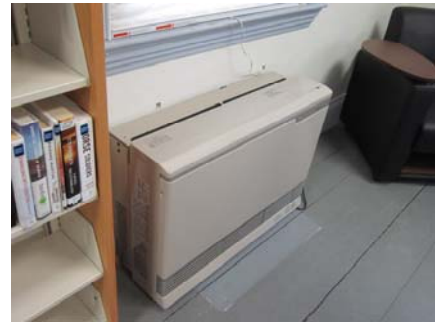
Figure 60 – Typical through-wall propane heater
