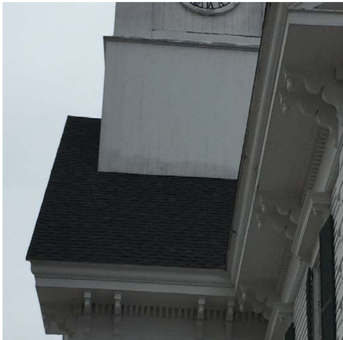
Figure 46 – Staining at tower connection to roof may be related to headwall flashing at double wall
