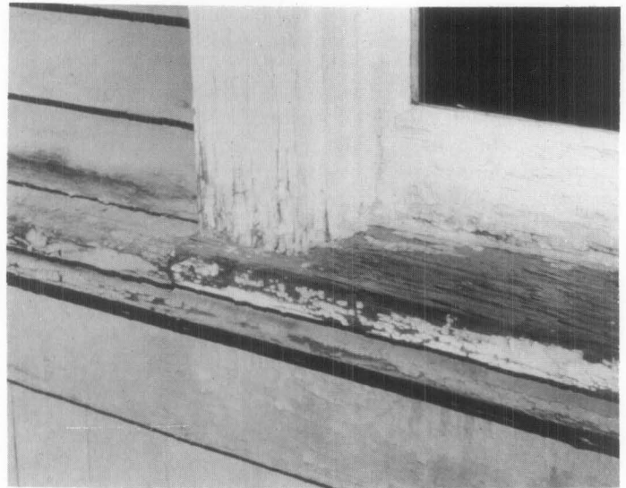
Fig. 4 Paint films wear unevenly depending on exposure and location. Exterior locations which are susceptible to accelerated deterioration are horizontal surfaces such as window sills. These and similar areas will require repainting more often than less vulnerable surfaces. In the case of this window sill where paint has peeled off and adjacent areas have cracked and alligatored, the paint should be totally removed. Prior to repainting, any weathered wood should be rejuvenated using a solution of 3 cups exterior varnish, 1 oz. paraffin wax, and mineral spirits/paint thinner/or turpentine to make 1 gallon. Liberal brush application should be made. This formula was tested over a 20-year period by the U.S. Department of Agriculture's Forest Products Laboratory and proved to be just as effective as water-repellent preservatives containing pentachlorophenol. After the surface has thoroughly dried (2-3 days of warm weather), the treated surface can be painted. A high quality oil-base primer followed by two top coats of a semi-gloss oil-enamel or latex-enamel paint is recommended. Photo: Baird M. Smith, AIA.
