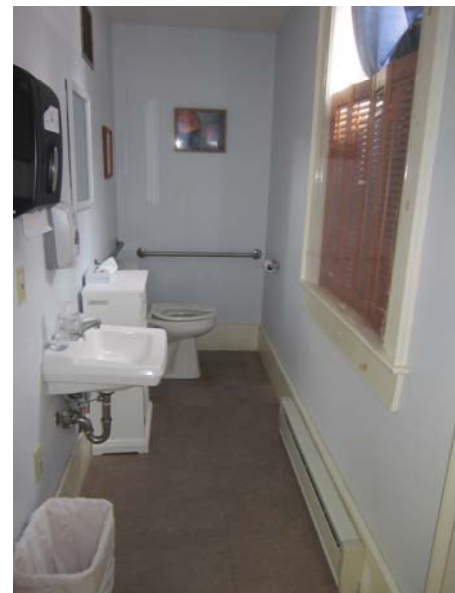
Figure 68– Existing restrooms are too narrow to meet ADA requirements for turning
