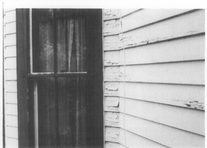
Fig. 8 Peeling to bare wood—one of the most common types of paint failure—is usually caused by an interior or exterior moisture problem. Photo: Anne E. Grimmer.
