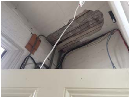
Figure 65 – Penetrations where pipes and wiring pass through corridor walls should be firestopped.
