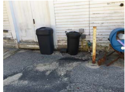
Figure 44 – Wood Clapboard siding (with timber sill behind it) in direct contact with pavement. Investigate for sill damage.
