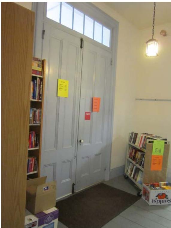
Four panel doors at Vestibule end or original Central Corridor match Exterior doors at other end now covered over at the interior but visible from the exterior
