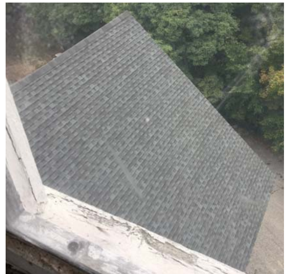
Figure 45 – Unvented architectural asphalt shingles on building main block (as seen from tower window)
