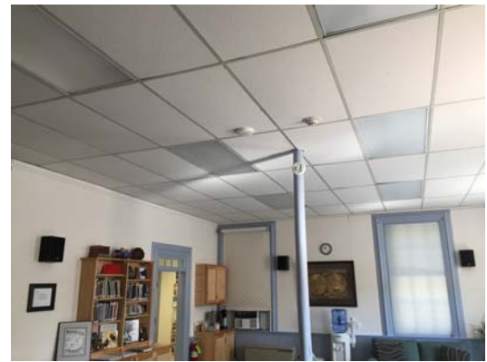
Figure 53– Lay-in acoustical tile ceiling throughout main level supports layer of fiberglass insulation
