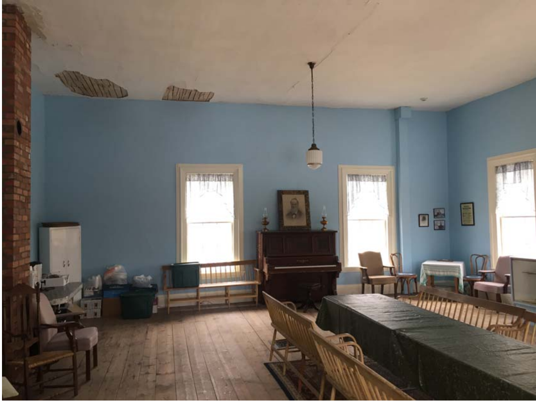
Mason's Meeting room showing Plaster Failures at Ceiling
