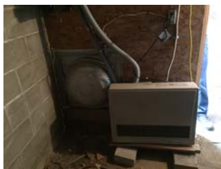
Figure 63– make modifications to basement space to control high humidity
