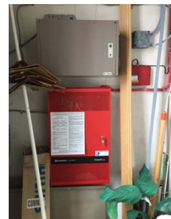
Figure 64 – Fire alarm panel located in Vestibule
