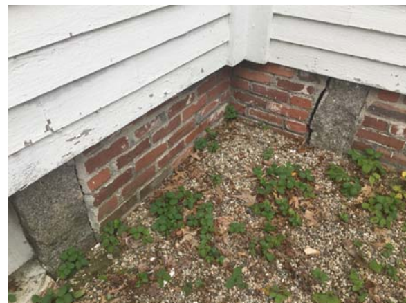
Figure 13: Unique Building Foundation – Granite posts at perimeter of building with non-structural brick infill masonry
